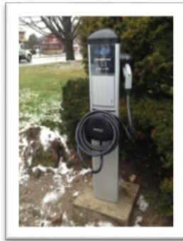
Montpelier, corner of State Street and Governor Aiken Avenue: Example of designated area after installation is complete
