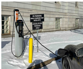
Level 2 Charging a Vehicle
