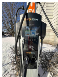
Level 2 EVSE Unit
