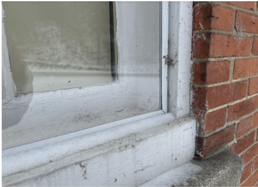
Detail photo of existing storm window. New storms will sit in the same opening.
