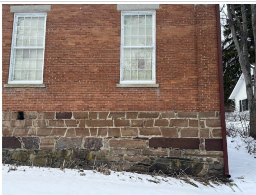
Proposed location of heat pump (will be placed on a stand close to the corner)
