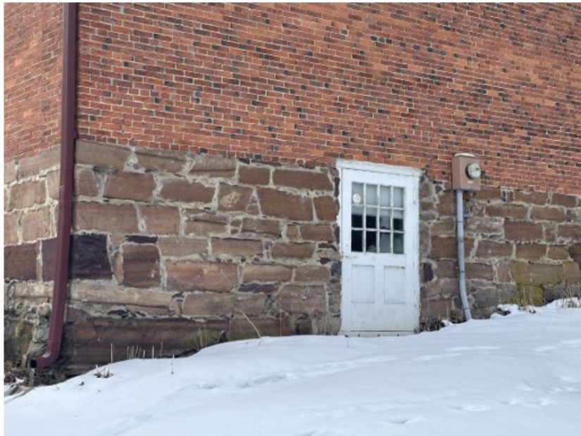
Existing basement door will be used to remove old boiler and install new boiler. Electrical service will remain in same spot (pole is just out of frame to the right)
