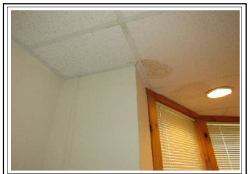
Ceiling spot water stain in lower level rec. room
