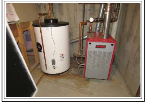
Furnace & hot water tank
