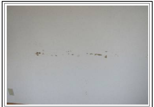
Damage to sheetrock
